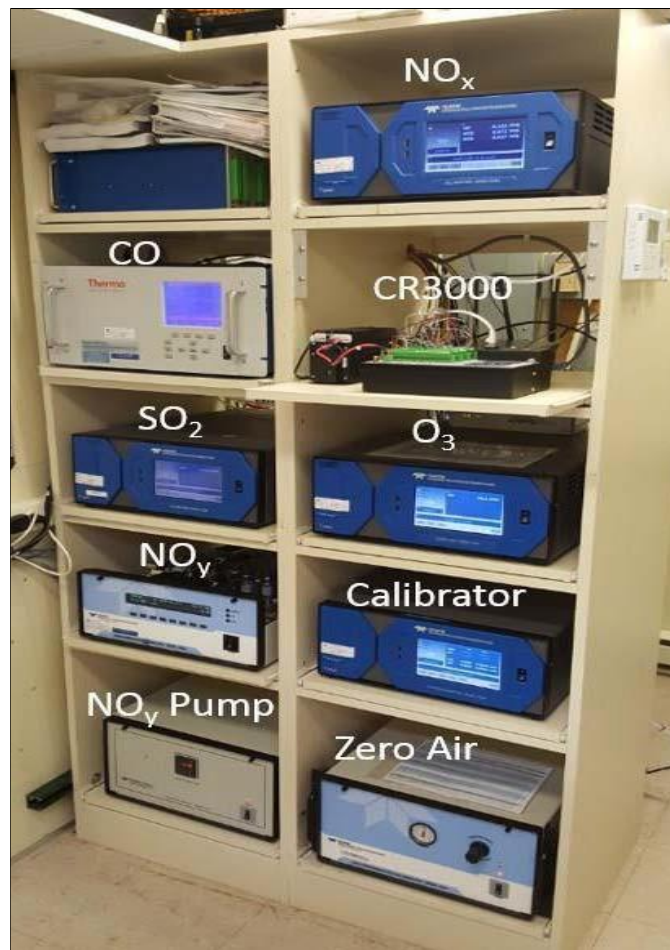
Figure 3. Configuration of Monitoring Equipment in the Instrument Rack
